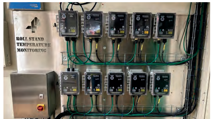
Recent multiple IE-Node installation at flour mill.
