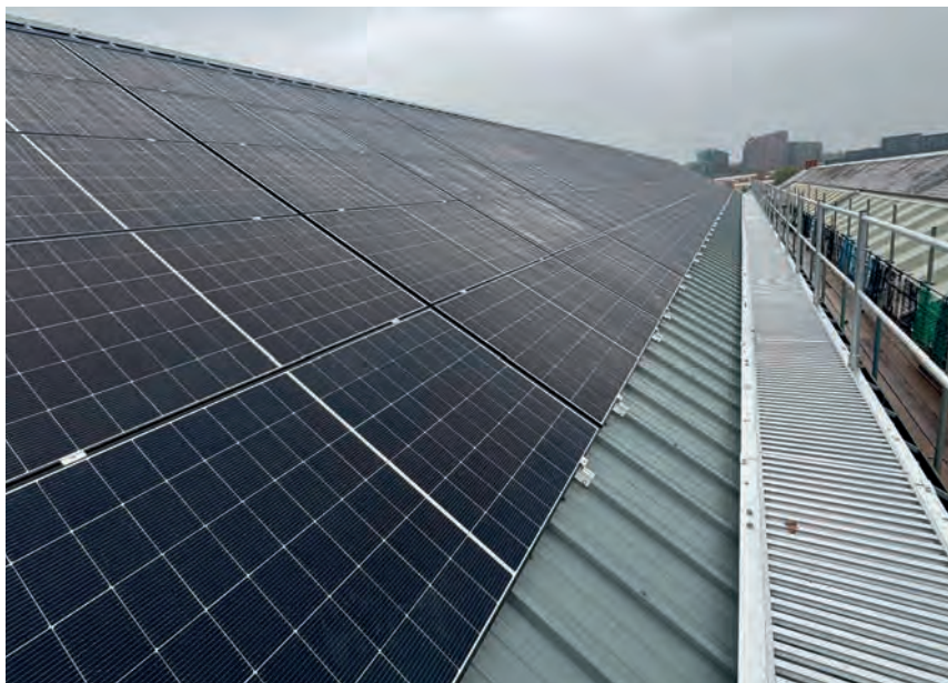
New solar PV installation at Braime headquarters, Leeds for energy utilisation by Braime Pressings.
